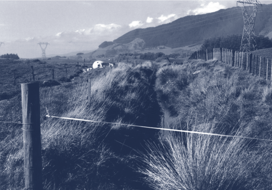
Good drain management will keep drain systems functioning effectively and efficiently. Photo: Greater Wellington.
