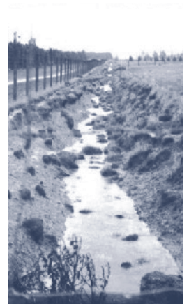
Stream bank erosion can be a source of sediment in drains.
